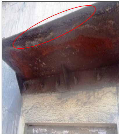
Cracks and seepage marks noted
